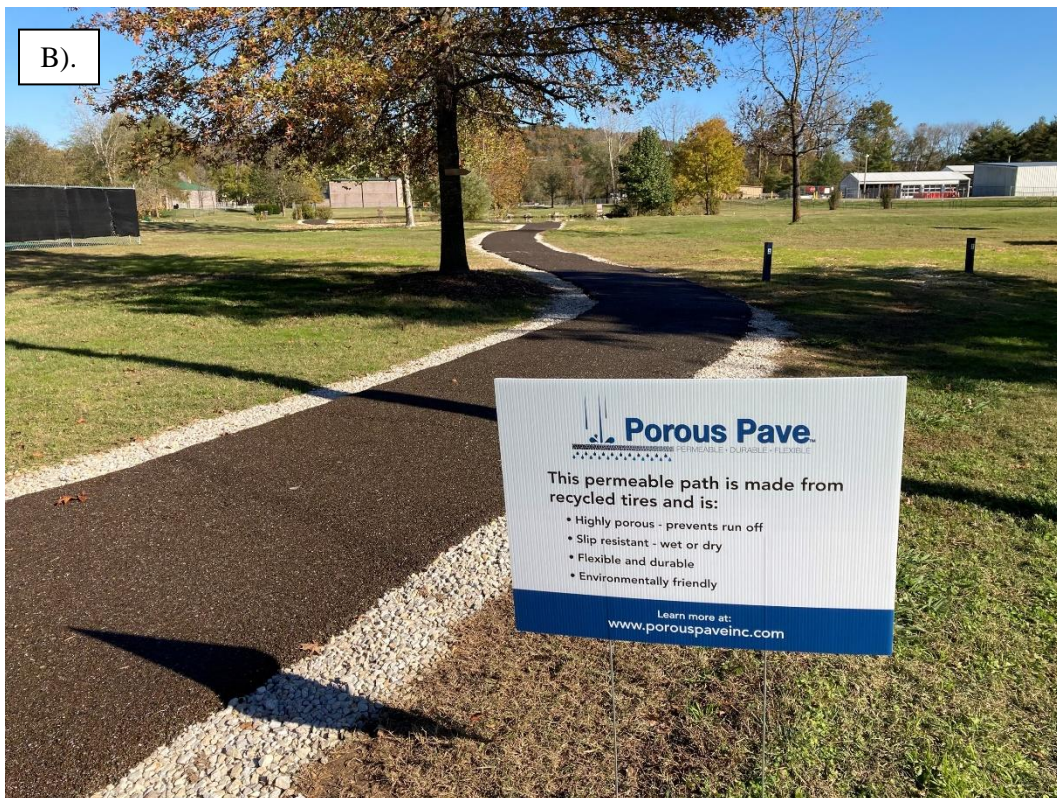
Figure 22. Porous Pavement Trail at Eiserman Park. A). Aerial view. B). Ground View. Photos from https://bransonmo.gov/890/Eiserman-Walking-Path .
